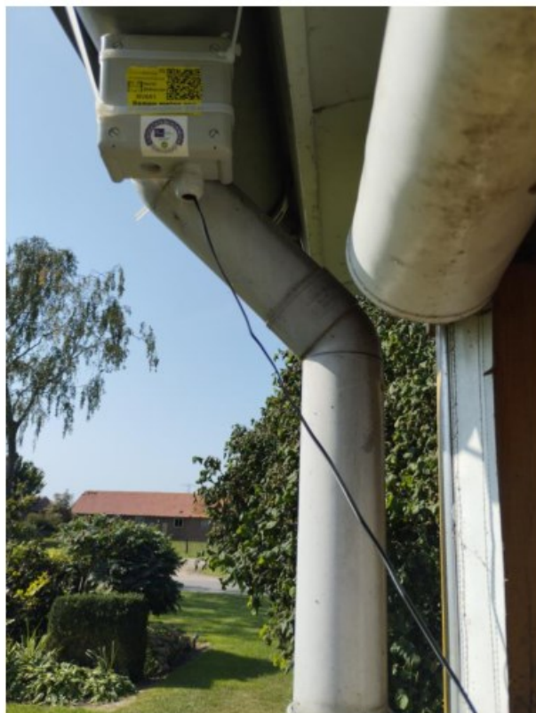
Fig.4: Example placement of a PM10 measuring sensor
